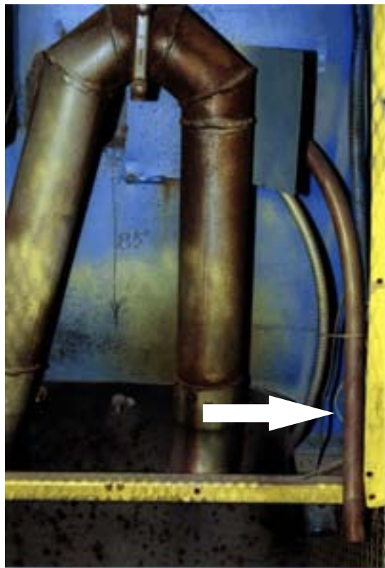
Photo 2. After end of the starboard-side main bilge pump discharge pipe
